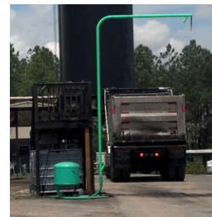
Drive Through Automatic Spray Arch
